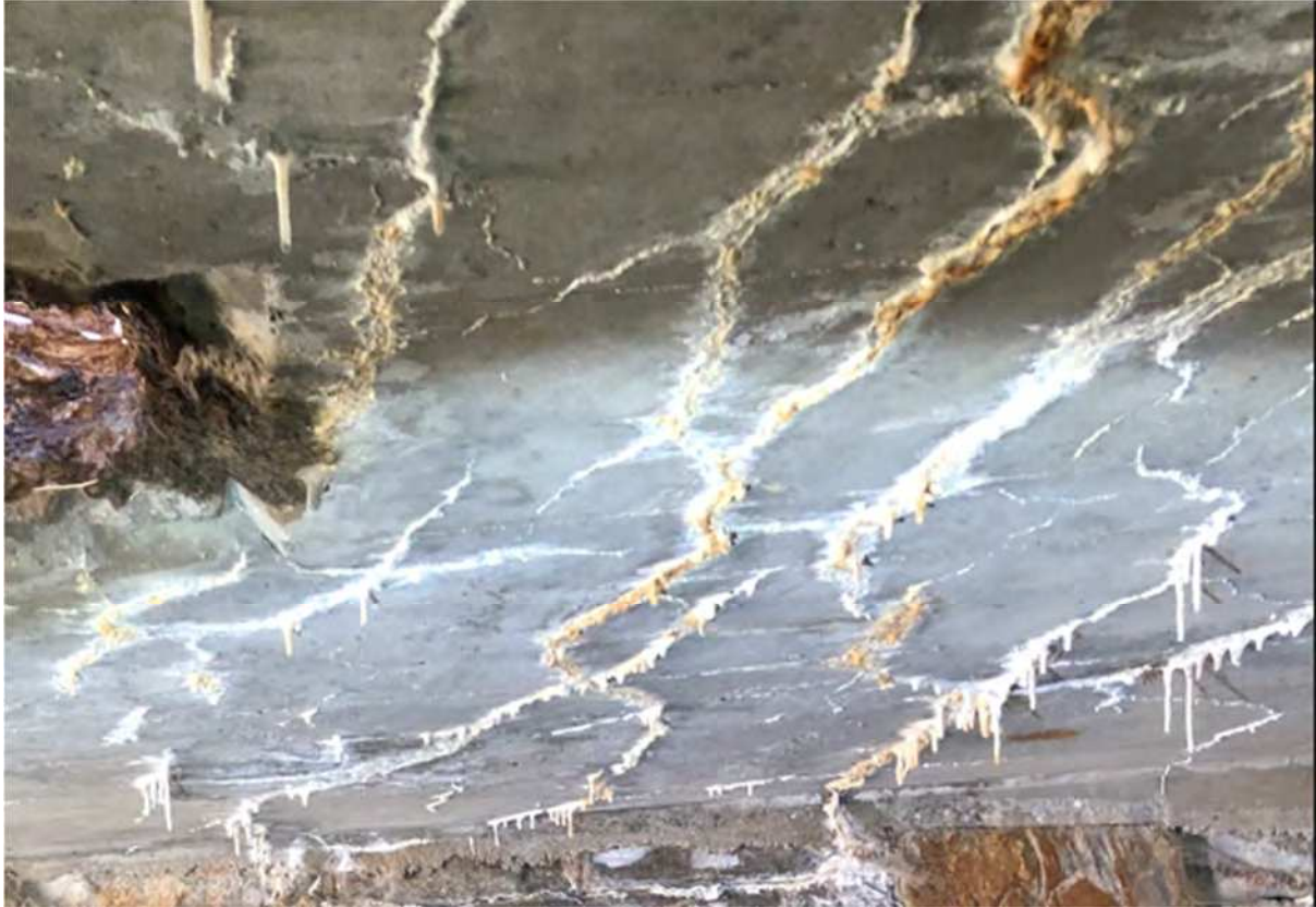
Figure 2-10: Efflorescence on the top slab of the culvert.
