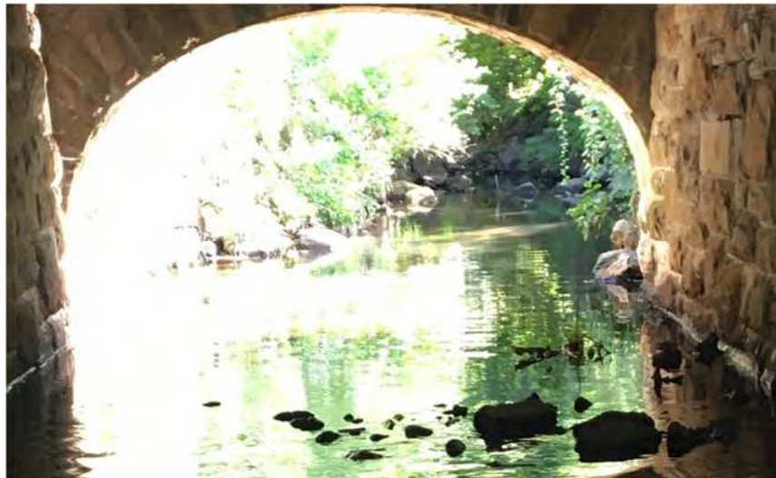
Figure 2-5: View of sediment accumulation and portion of branch caught at inlet.
