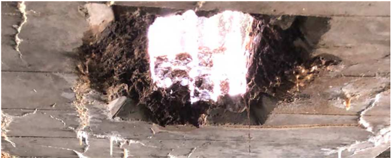
Figure 2-13: Abrasion and surface damage on the top slab at the drainage holes.
