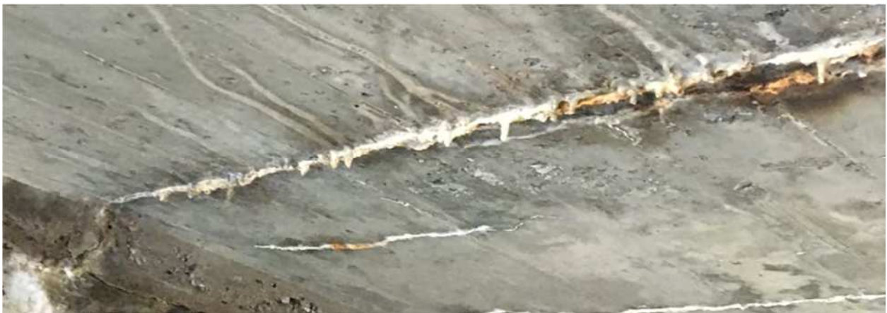
Figure 2-18: Joint on top slab of culvert with heavy efflorescence but not cracking.
