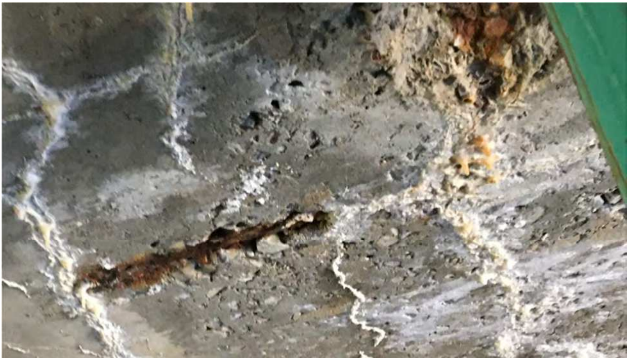
Figure 2-12: Visible rebar and segregation on the top slab.
