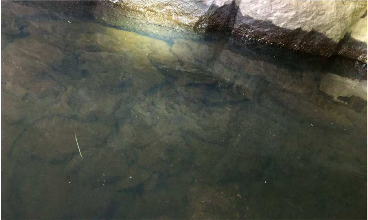
Figure 2-8: Previously buried section of culvert unearthed by scour.
