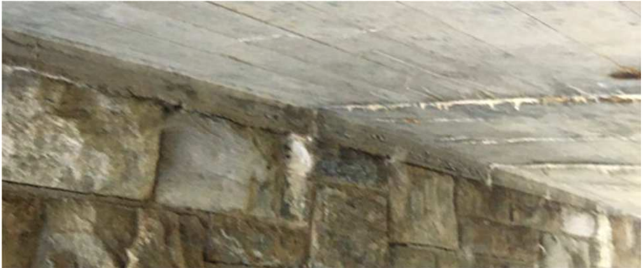
Figure 2-17: Joint separation where the top slab meets the masonry wall.
