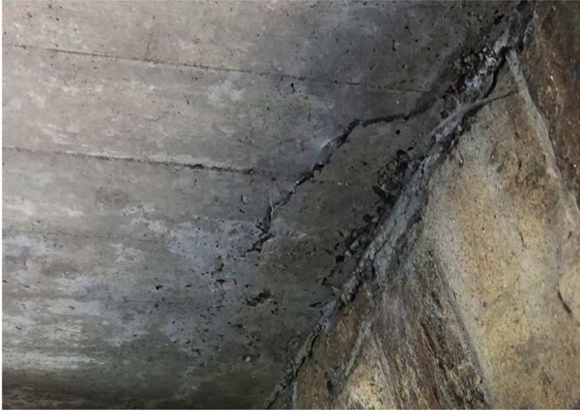
Figure 2-11: Delamination at the inlet of the culvert on the top slab.
