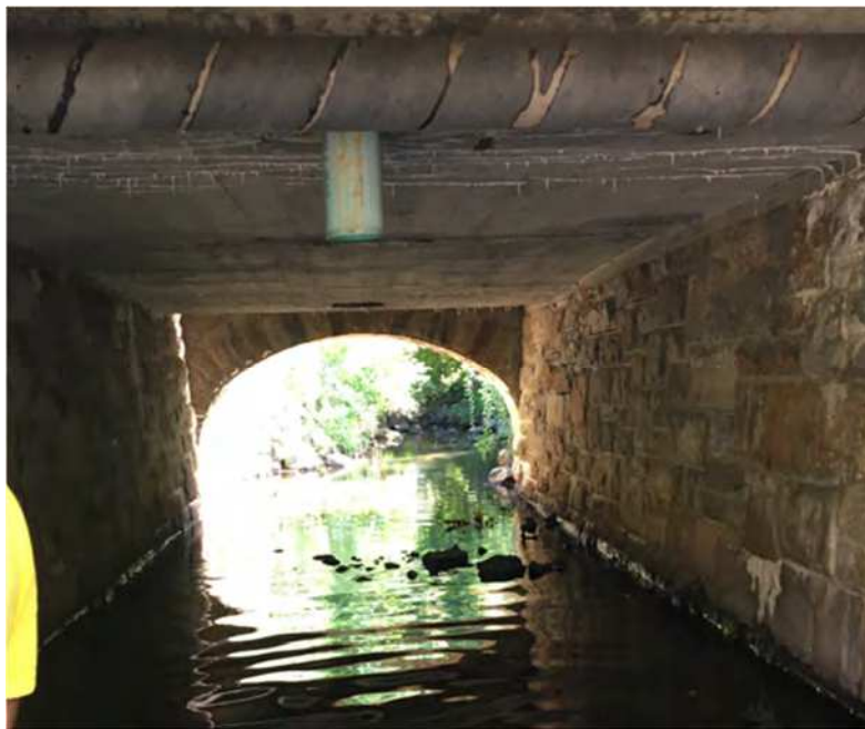
Figure 1-3: View of the inside of the culvert. Walls are stone masonry blocks and the top slab is reinforced concrete.
