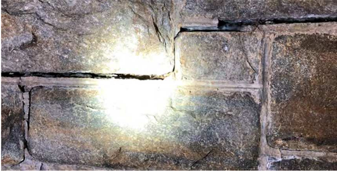
Figure 2-14: Separation between the masonry blocks and mortar joints.
