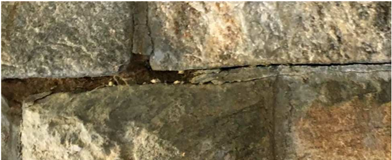
Figure 2-15: Missing mortar between masonry blocks; note that differences between the outer and inner mortar.
