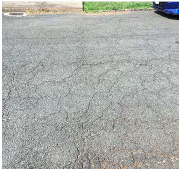
Figure 2-1: Transverse cracks forming at the structure and approach roadway intersection.
