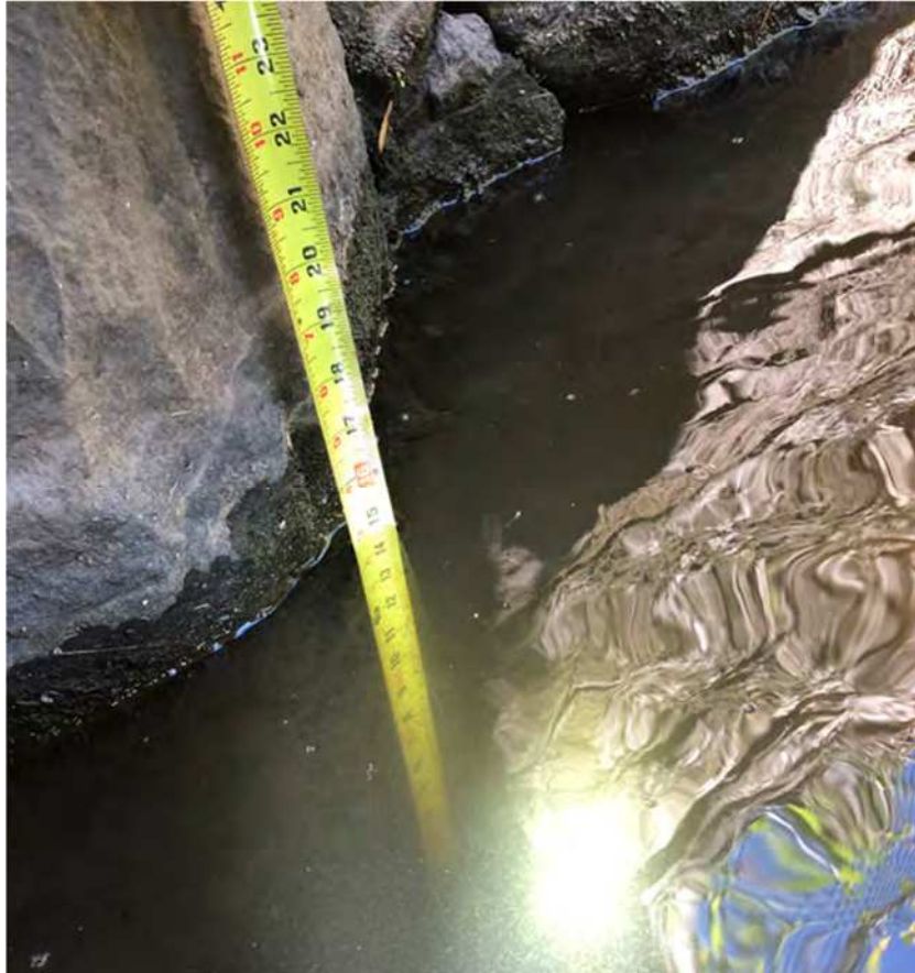
Figure 2-7: Depth to top of footing at end section's scour hole.
