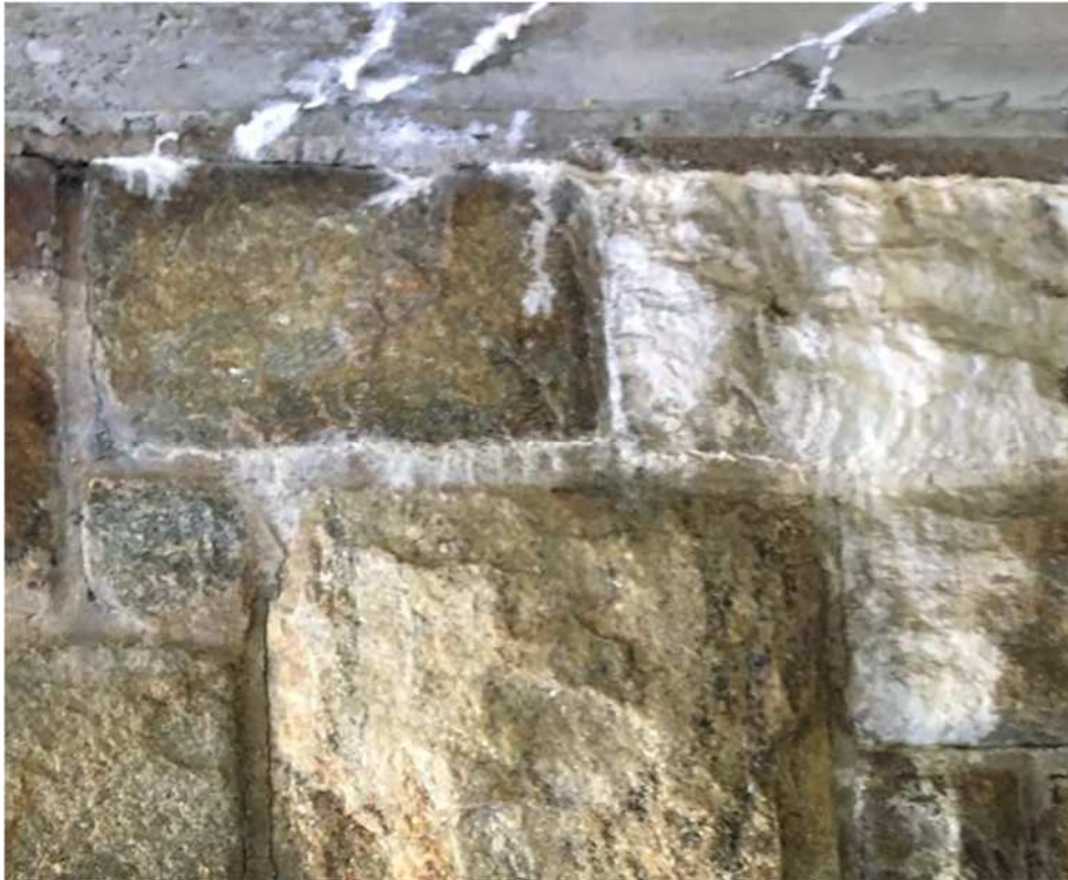
Figure 2-16: Isolated efflorescence on the masonry.
