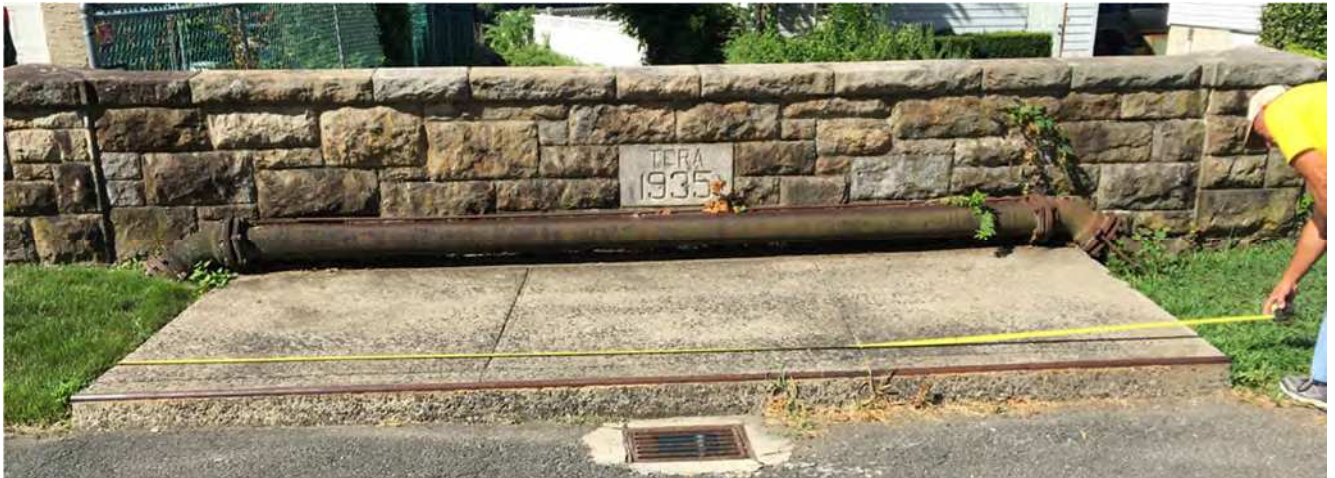
Figure 1-7: Sidewalk and stone masonry block parapet over the culvert. Note utilities and drainage over the culvert.
