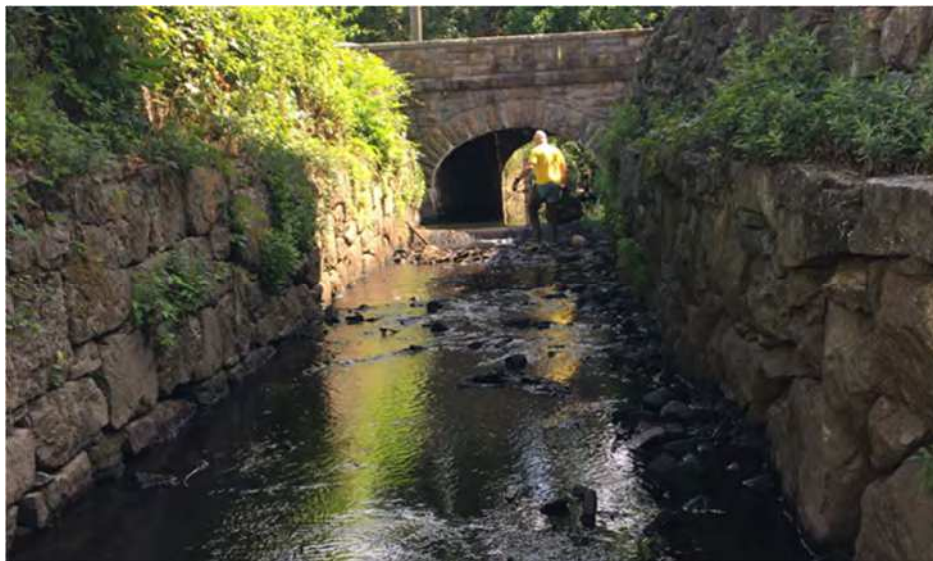
Figure 1-5: In-line walls guiding Beaver Swamp Brook. Photo taken downstream looking upstream (looking at outlet).
