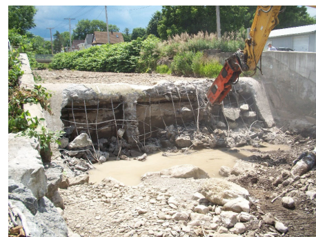
Top Right: Remington Arms Dam, Ilion, NY, before construction, 2019 Bottom Right: Remington Arms Dam, Ilion, NY, during construction, 2020
