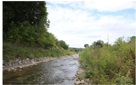
Top Right: Steele Creek, Ilion, NY, during construction, 2020 Bottom Right: Steele Creek, Ilion, NY, after construction, 2021
