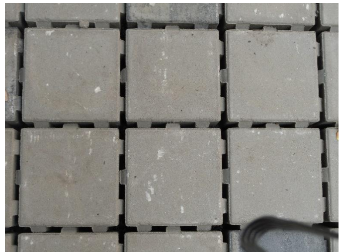
Void space between individual pavers allows water and air to infiltrate
