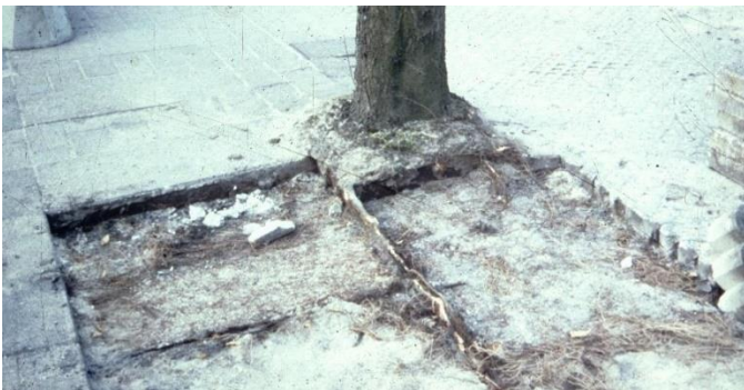
With paving removed, it is easy to see how this tree's roots took advantage of the weak points in the pavement. While the tree survived, the expanding roots caused the pavement to fail.
