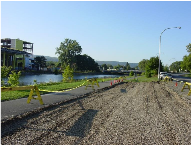
CU Structural Soil® was used as a 2' deep base course for the entire parking lot
