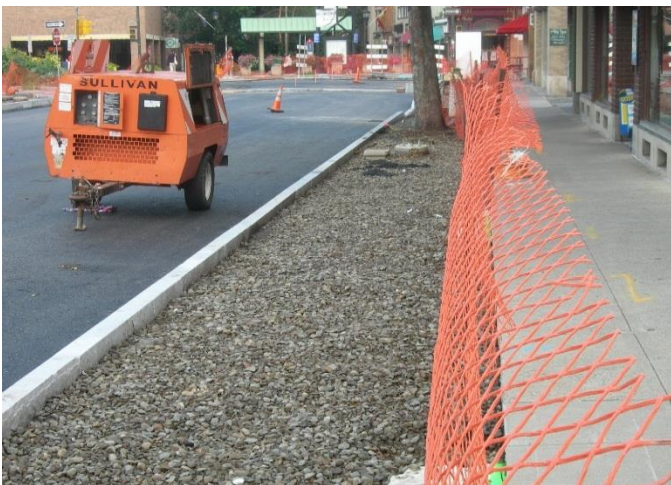
Installation of the new sidewalk on a base of CU-Soil®. This picture also shows an existing mature tree
