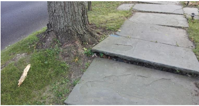
Tree roots heaving pavement
