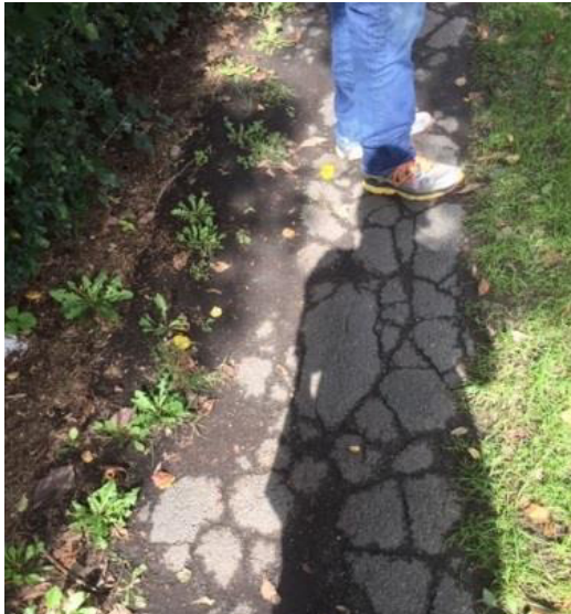
Figure 133: A section of the sidewalk along N. Barry Ave (photo by Shannon Purdy)
