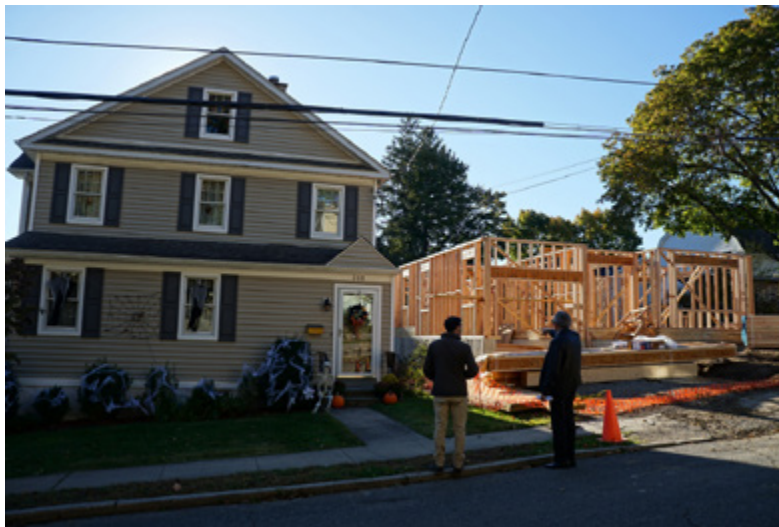
Figure 71: A new house is being constructed as a result of a tear down
