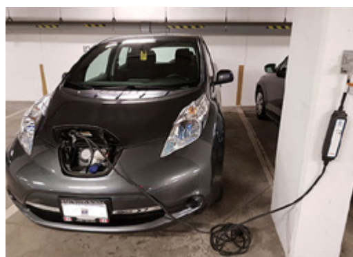
Figure 47: An electric vehicle is being recharged inside the parking structure of an apartment building.
