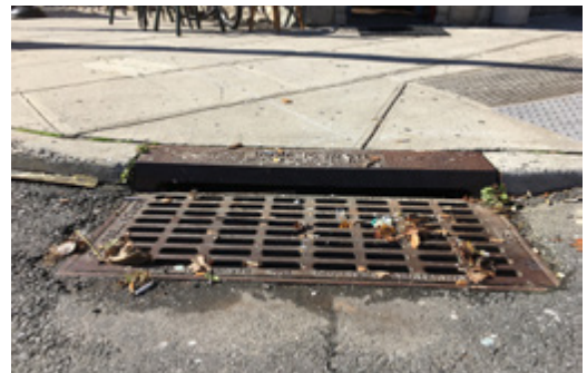
Figure 135: A storm drain
