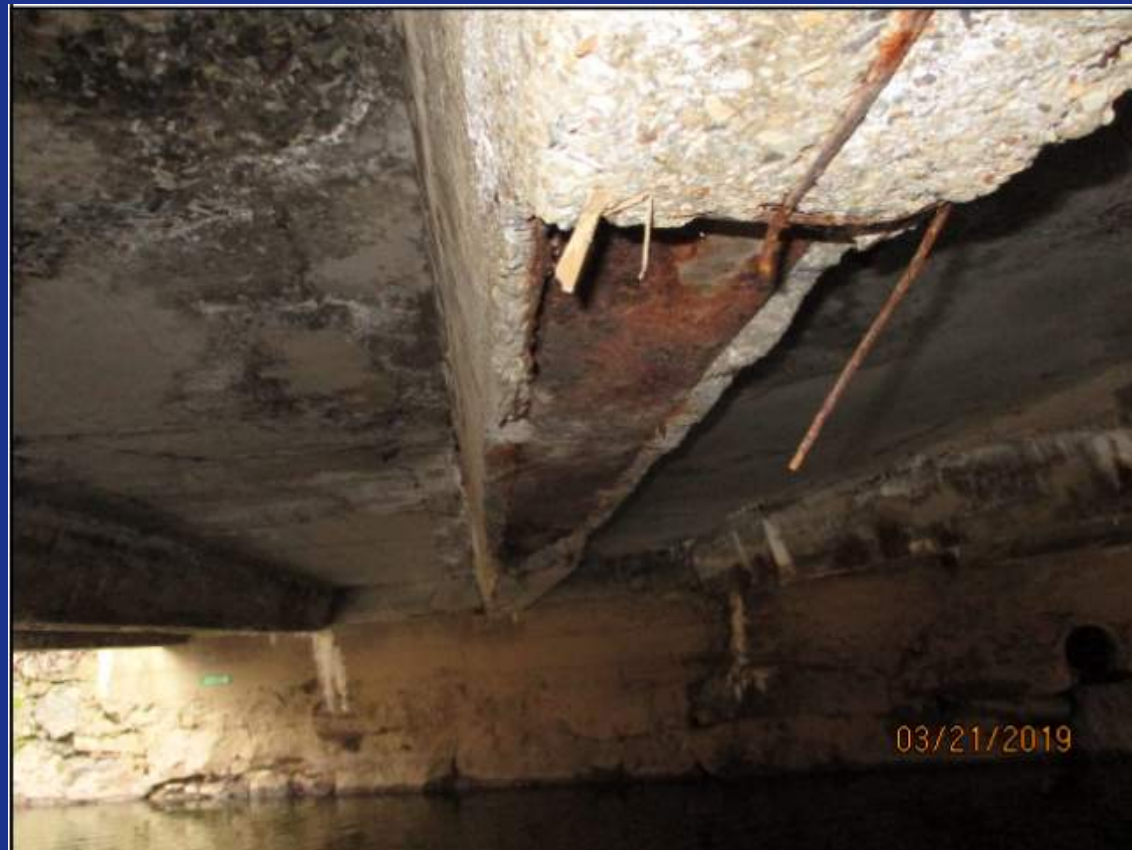
Deteriorated Concrete Encasement (photo from 2019 Inspection Report)
